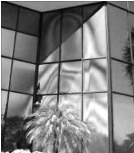
"Virgin Mary" sprinkler stain on a building
